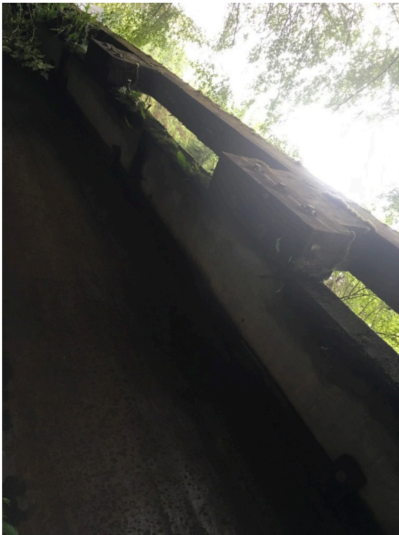
Missing tie clip
